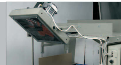
5 Cooling fan after shrink tunnel
